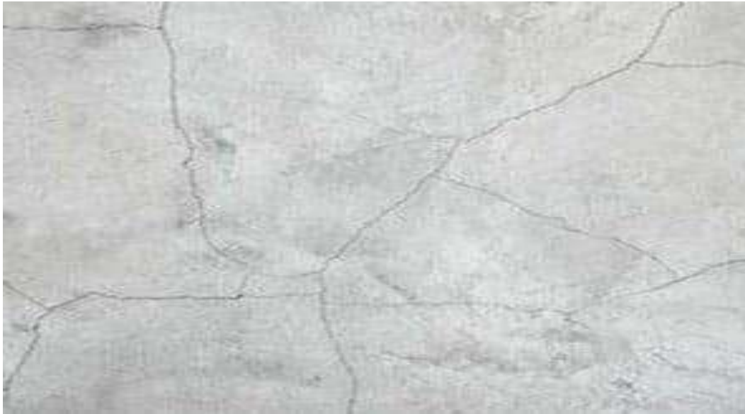
Fig 2.4 Thermal cracking of concrete slab
