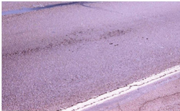
Fig.3: High Severity of Raveling Distress in Flexible Pavement [12]
