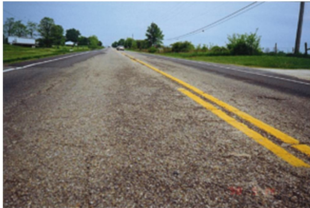
Fig.2: Medium Severity of Raveling Distress in Flexible Pavement [12]
