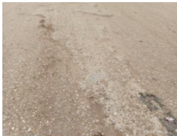
Fig.15: Medium severity of Bleeding distress on Forestry road pavement
