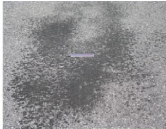
Fig.14: High Severity of Patching distress on Forestry flexible road pavement
