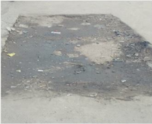
Fig.17: Failed section on Forestry road pavement
