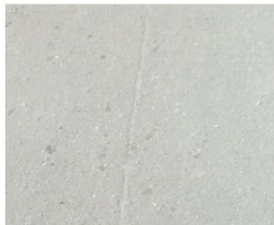
Fig. 16: Low severity of longitudinal crack distress on Forestry road pavement
