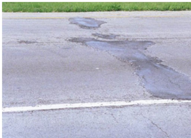
Fig.7: High Severity of Patching Distress in Flexible Pavement [12]
