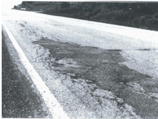
Fig.6: High Severity of Patching Distress in Flexible Pavement [12]
