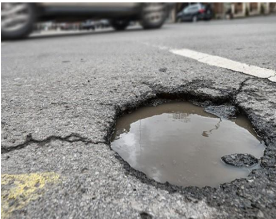
Plate 4: Potholes Caused by High Temperatures (Source: Field Survey, 2025).
