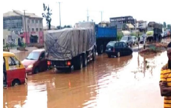
Plate1: Benin – Asaba Road failed portion due to flooding (source: Field survey, 2025).
